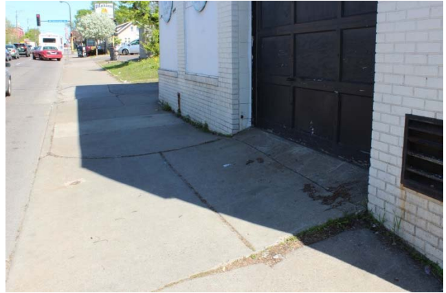
Figure 6. Driveway Apron Grades Limit Accessibility
