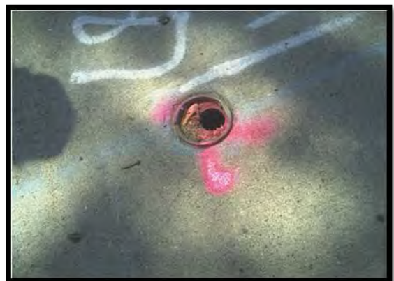
Water Gate Valve
