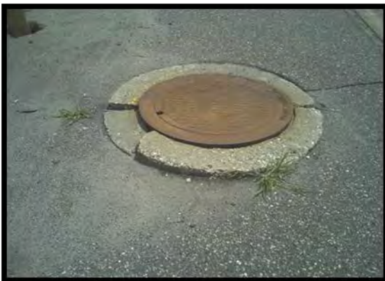
Traffic Signal Handhole
