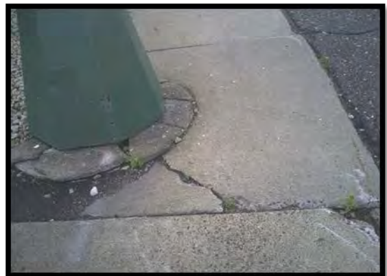
Traffic Signal Pole
