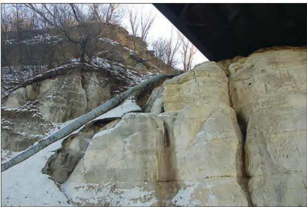
Figure 7.8b — Erosion of St. Peter Sandstone Downstream Side of Highway 5 Bridge
