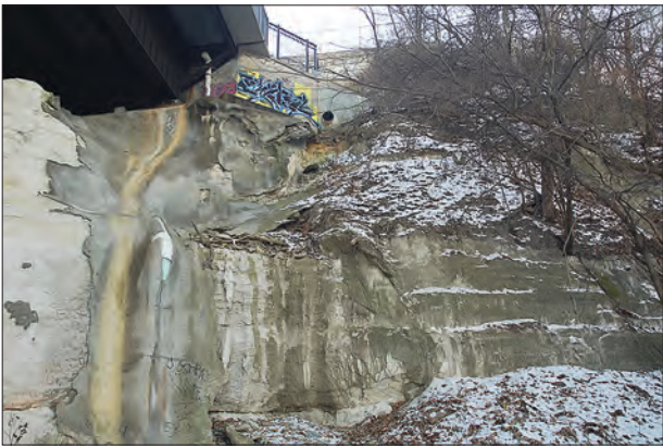
Figure 7.8a — Erosion of St. Peter Sandstone Near Infrastructure
