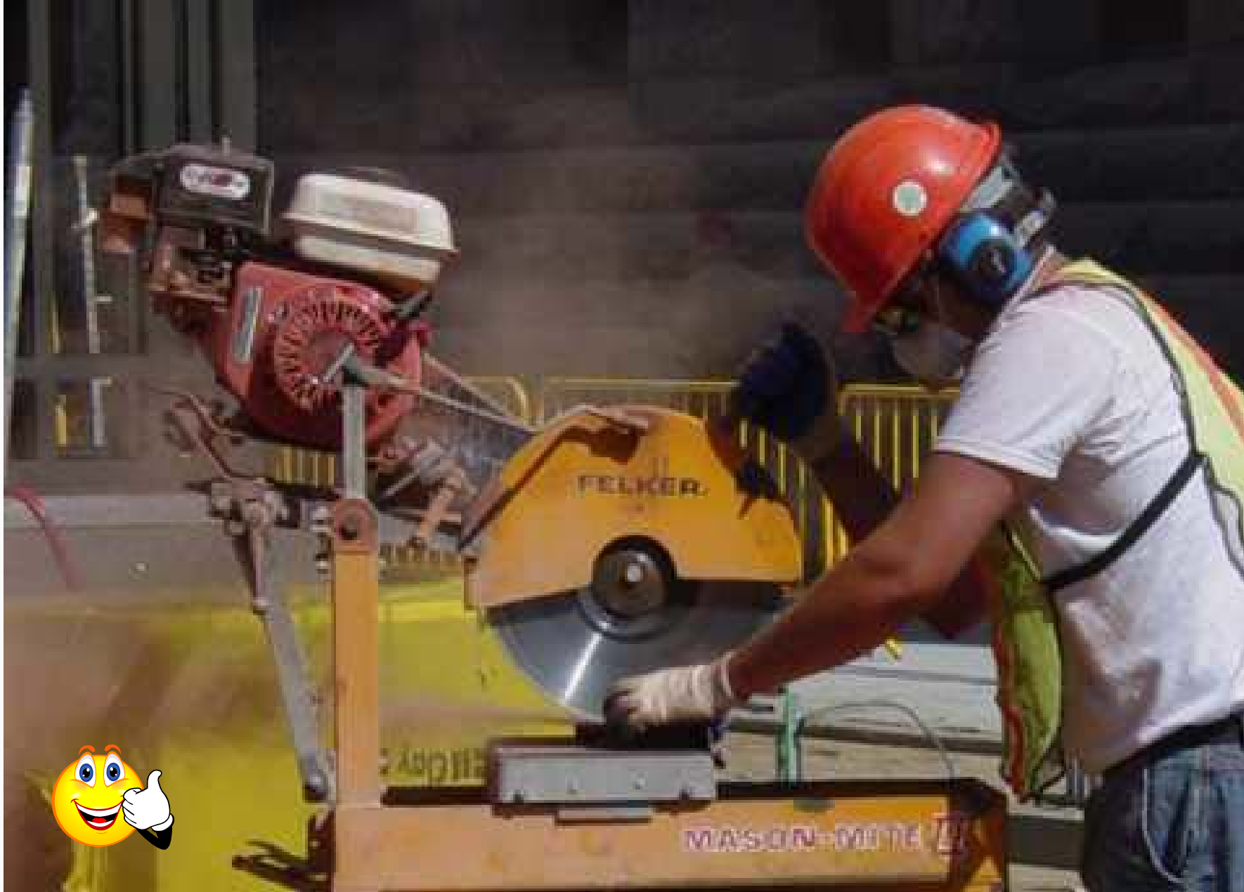
Worker wearing personal protective equipment suited to the hazards of the work.
