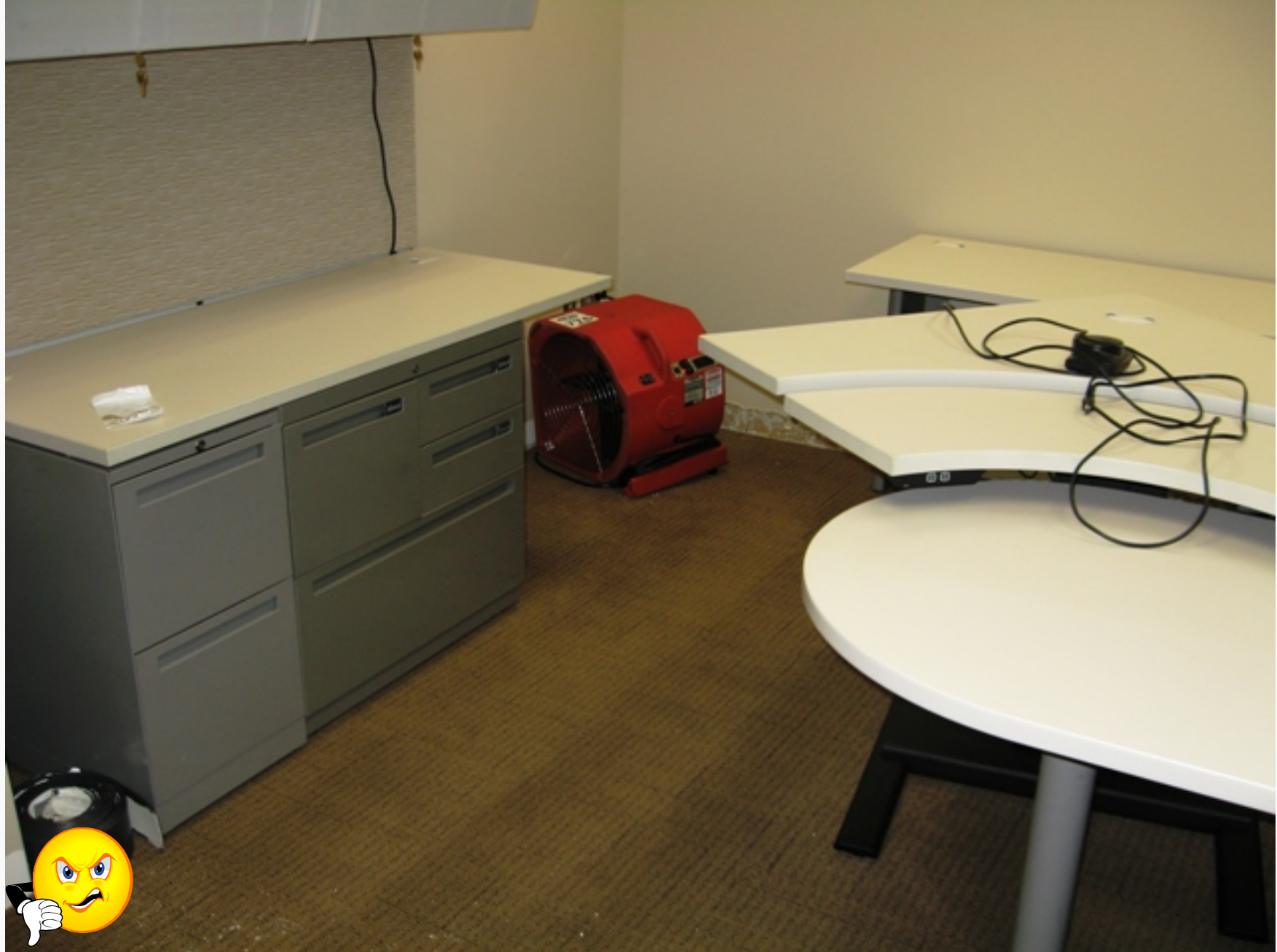
Water damage is very disruptive and costly.
