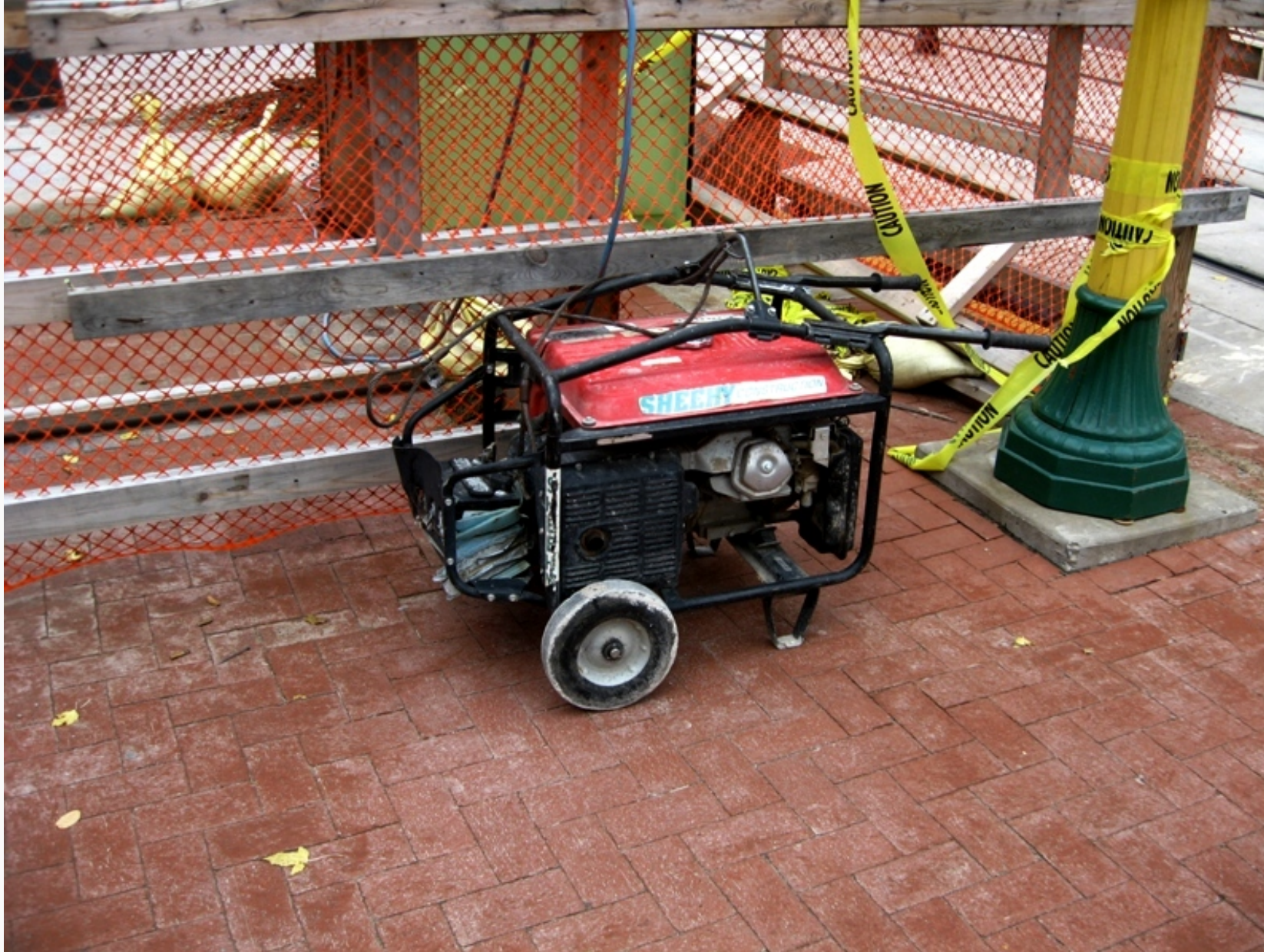
Engines and pneumatic tools may create disruptive noise conditions for facility occupants.
