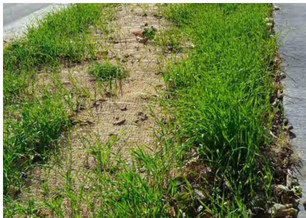
Native seeding accompanied by an erosion control blanket and growing cover crop.
