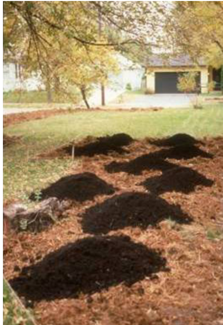
Soils amendments should be fully decomposed and meet MN DOT standard specifications.
